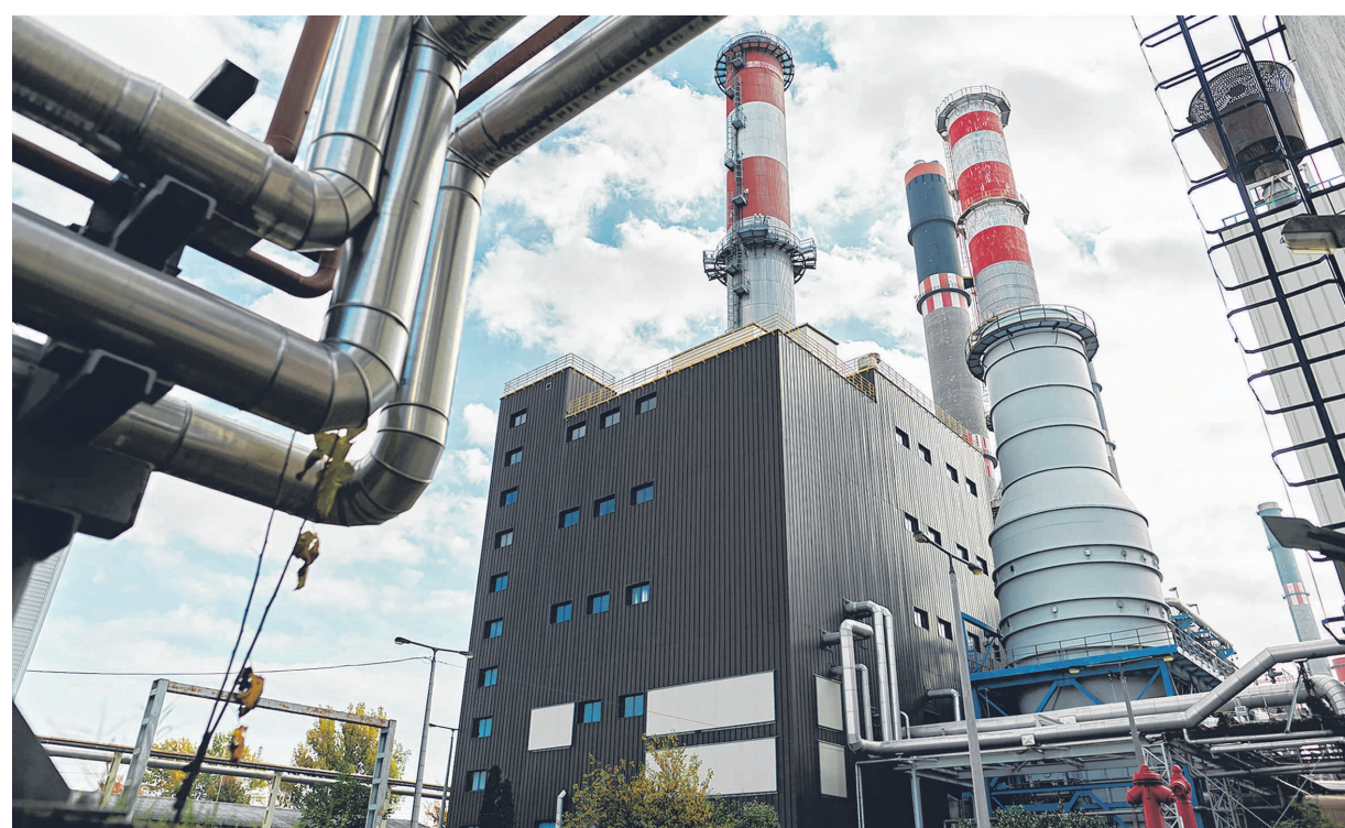
Switzerland-based European energy company MET Group is the majority owner of Hungary's largest gas-fired power plant, the 794 MW Dunamenti Power Plant. PHOTO: KEPPEL INFRASTRUCTURE
